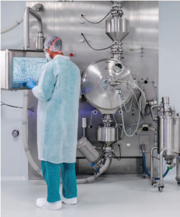
Hovione has installed state-of-the-art Continuous Tableting equipment
